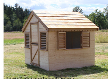
Install the scaloped trim. Start with the angled pieces setting them on the edge of the roof panels.
