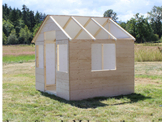
Set the roof panels. Make sure the top is exactly on the ridge so both panels will close tight.
